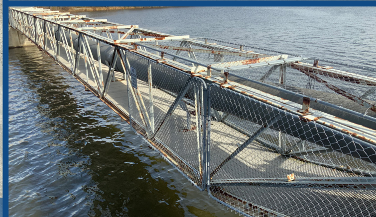
Steel truss supporting water main. Water main will be maintained during construction.
