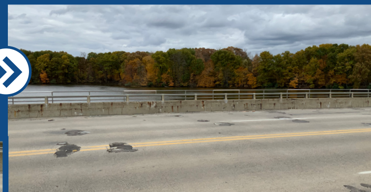
Spalled areas on the deck have been patched with cold patch, allowing water and salt to sit in these locations further deteriorating the deck. The deck and superstructure will be replaced.
