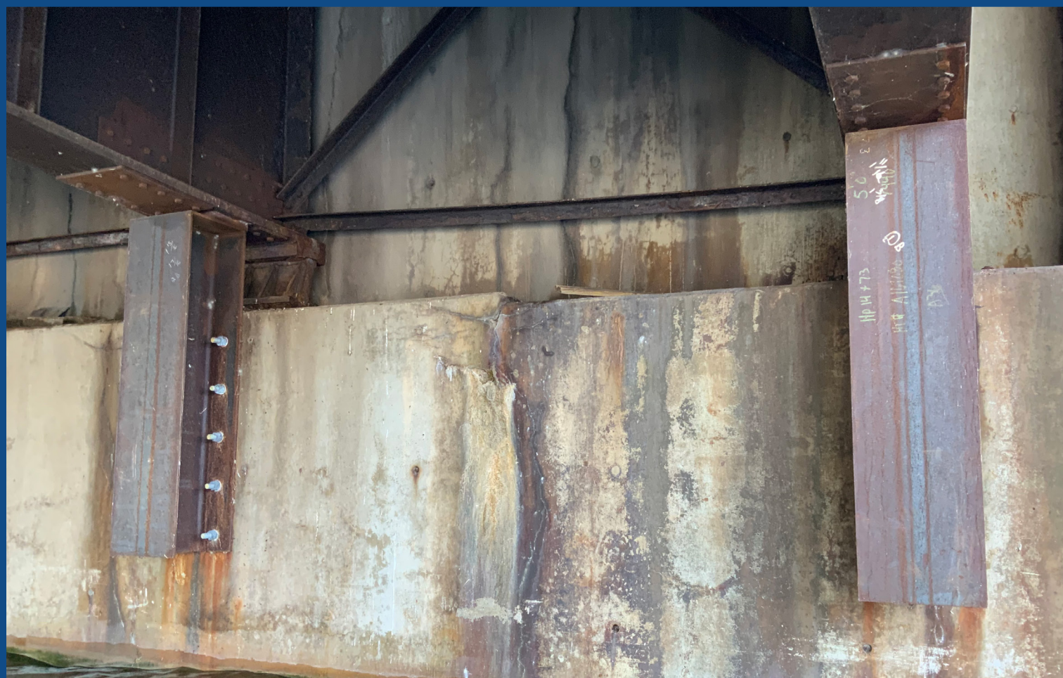
Temporary steel supports under each beam, these steel supports allow the structure to be posted at 30 tons. The new superstructure will restore full capacity to the bridge.
