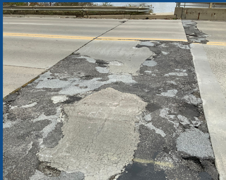
The approach slab has spalled and has been patched with cold patch material, increasing the impact loading on the bridge. The approaches will be replaced, creating a seamless transition to the bridge deck.
