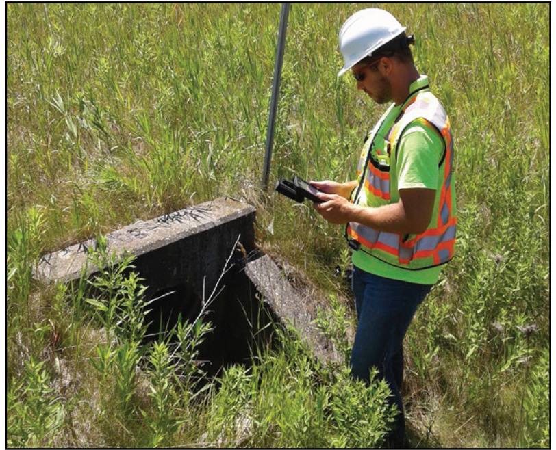
Above, ROWE's Bob Church records data about a culvert off US-131 near Standwood with a Trimble R-1 GPS antenna connected via Bluetooth to a Samsung tablet.
